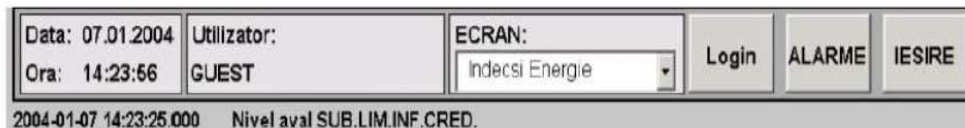
Figure 2. The control bar of the application at a SCADA system from a hydro power plant
