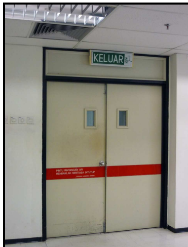
Figure 2. An exit sign above the fire door
