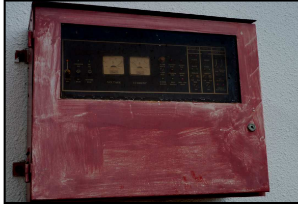
Figure 4. The Carbon Dioxide system control panel
