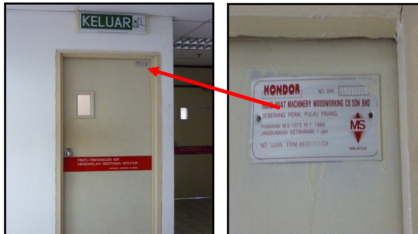
Figure 3. The fire door and the certification of the fire door
