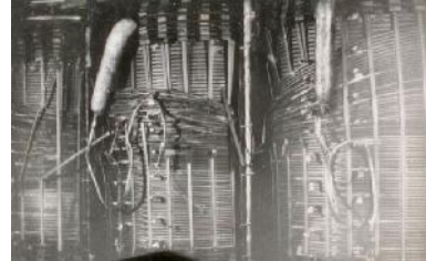
Figure 13. Fault of a transformer of 40 MVA, 110/6,6 kV [7]
