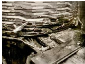
Figure 5. Fault of a transformer 16 MVA; 10/6,3 kV [7]
