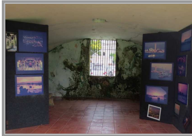
Figure 24. Dampness problem occurred in one of the cell rooms
