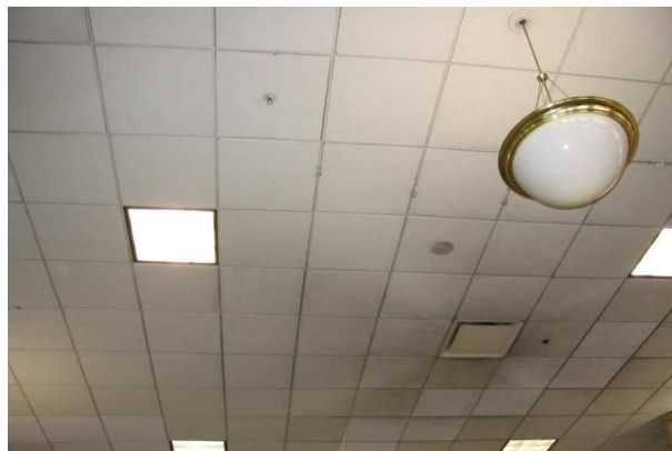
Figure 2. Ceiling in Baling Bayu Engineering shown the loose sheet of ceiling
