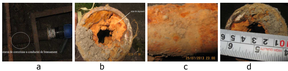
Figure 2. The wear and clogging status of cold water supply system a-external corrosion degree inside the branching pipe, b- clogging degree of the branching valve, c- external corrosion degree inside the pipe distribution, d- clogging degree of the distribution pipes
