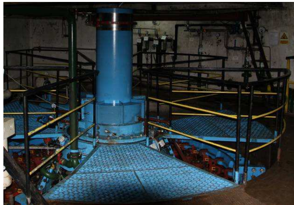
Figure 1. Turbine shaft, turbine bearing and wicket gates
