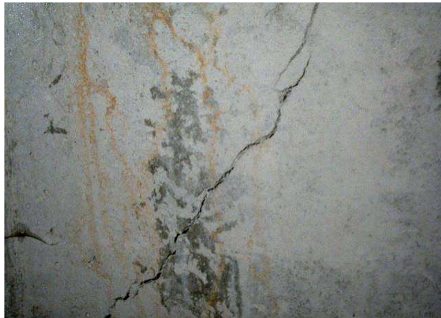
Figure 4. Minor cracks happened at internal section of the building
