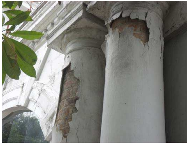
Figure 1. Loose plaster at the external column section
