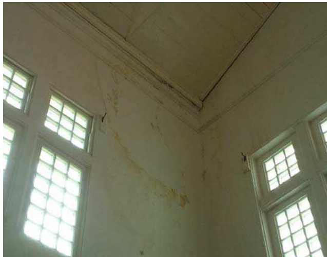
Figure 5. Sign of leakage in the ceiling
