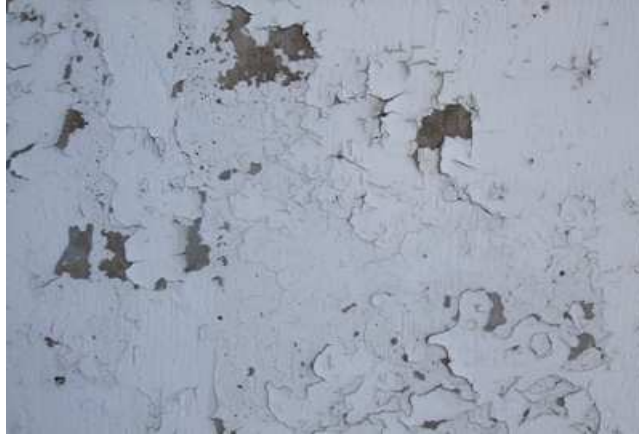
Figure 3. Paint peeling problem occurred at external section of the building
