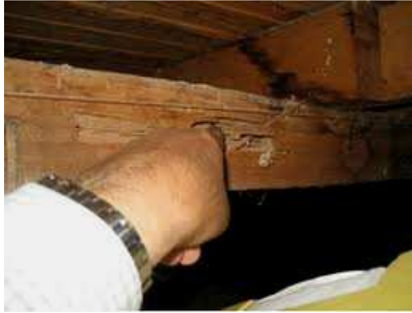
Figure 6. Extensive termite damage
