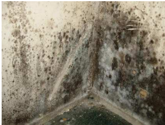
Figure 7. Dampness problem on interior wall surface
