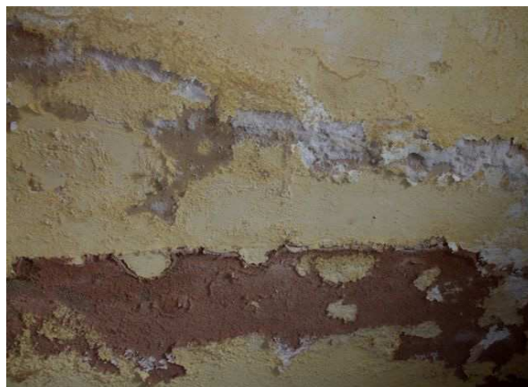
Figure 4. Salt attach to brickwork
