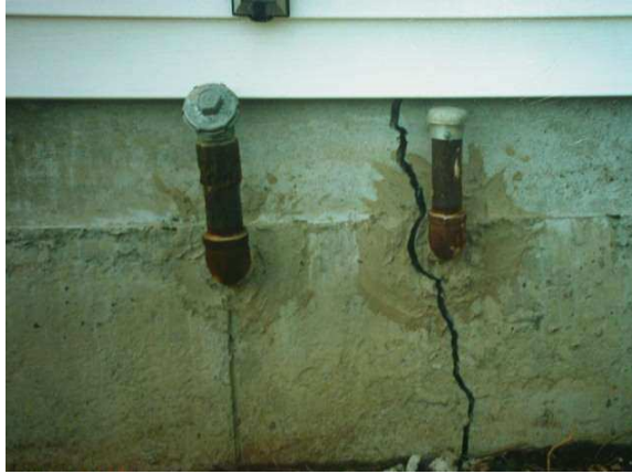
Figure 2. A significant settlement crack
