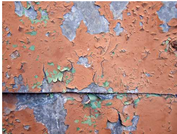
Figure 5. Peeling paint from wall surface
