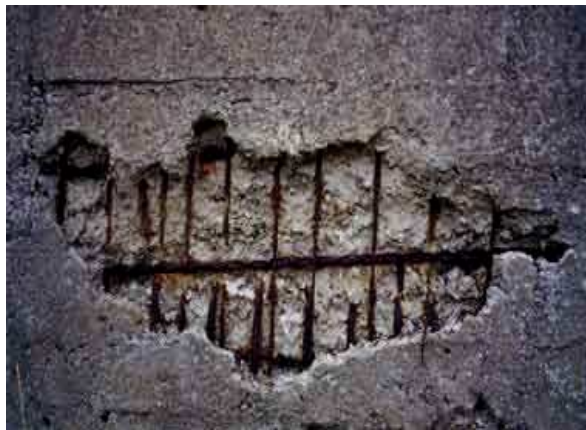
Figure 3. Concrete spall exposing the rebar
