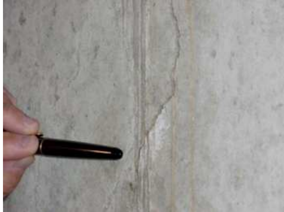
Figure 1. Shrinkage cracks appear on wall
