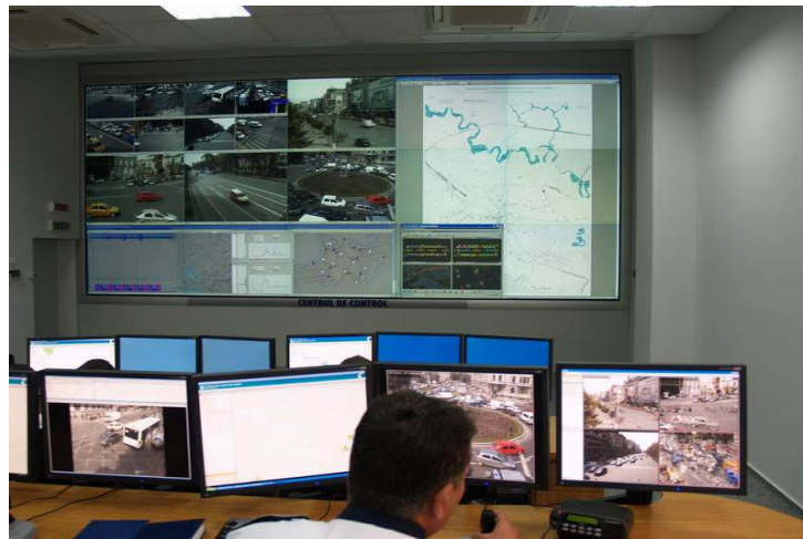
Figure 16. The BTMS Control center
